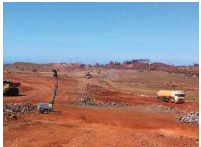
Earthworks being conducted by NRW at the Rio Tinto Cape Lambert expansion
